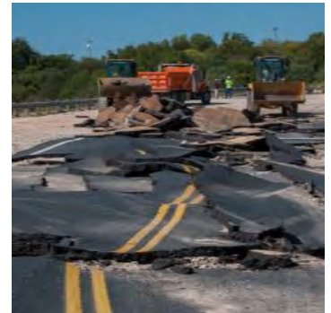
The Halloween Flood of 2013 caused damage to Austin roads that had to be addressed immediately.
