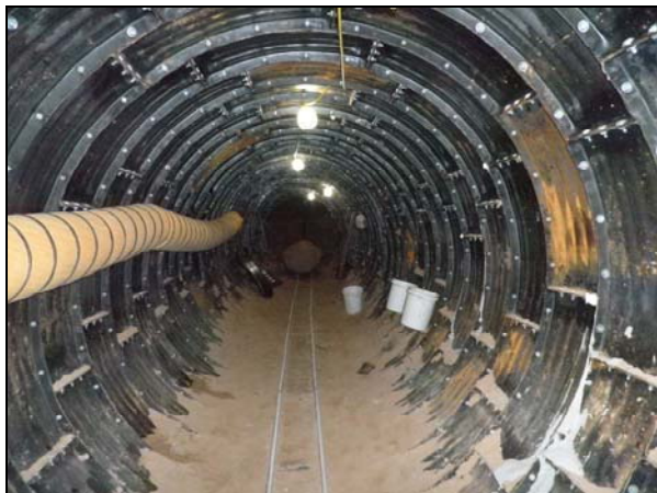
Tunneling operation to install a new 72-inch RCP under the CapMetro Redline as part of the East 4 th /Pedernales stormdrain improvement project.
