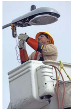
Dark Sky streetlight infrastructure upgrades | p. 195
