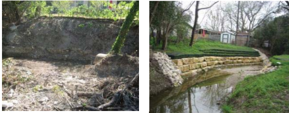
East Bouldin Creek at Wilson St Culvert Outfall Bank Stabilization (before and after)
