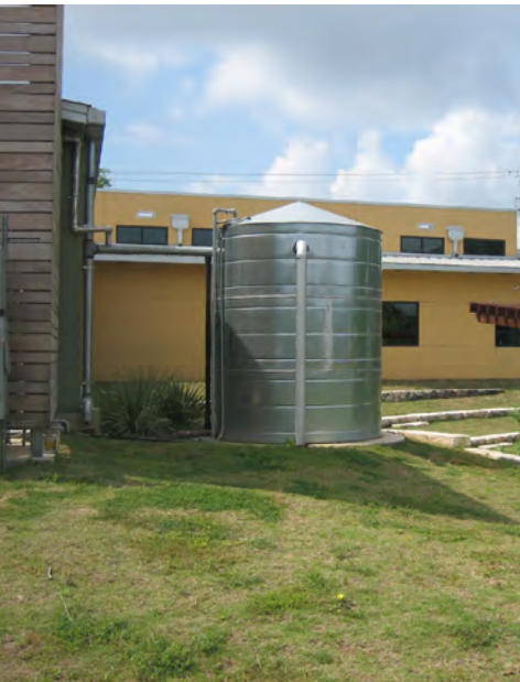
The recently constructed Twin Oaks Library in the Bouldin neighborhood incorporates many sustainable design elements including water collection, water harvesting, and solar power.
