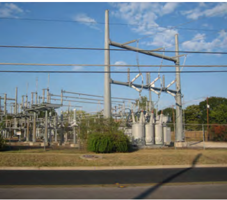
A transformer station in Northeast Austin.
