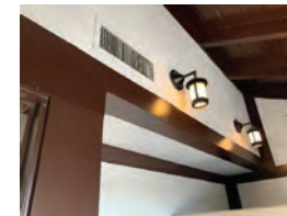
Figure 2: Bathroom Heating Supply and Return
