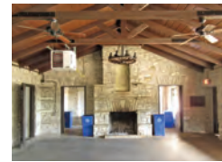
View to the north of the Main Room. The original window opening on this wall was converted to door openings to access the restroom addition in 1996.
