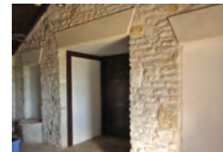
The restroom addition uses similar stone wall construction, with smooth stone headers at the openings.
