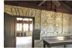
View to the east in the Kitchen. Surface-mounted conduit and electrical device boxes provide power for catering use.
