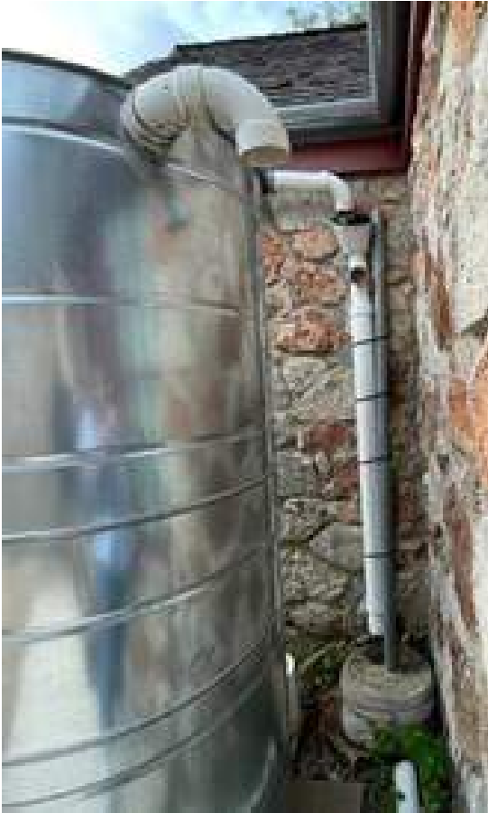
Rainwater Treatment of Caretaker's Cottage
