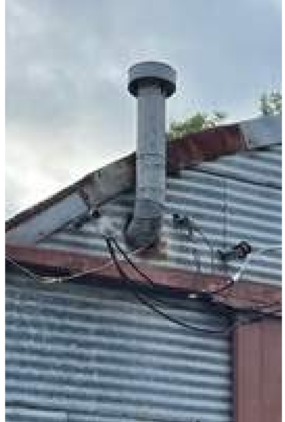
Ventilation of Quonset Hut
